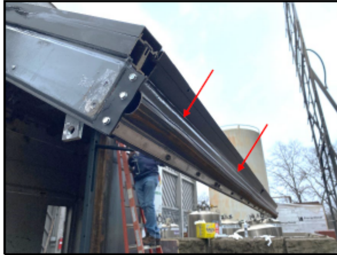
Photo No. 19 Exterior View of Operable Steel Frame at Sill with New Horizontal Gasket and Aluminum Angle
